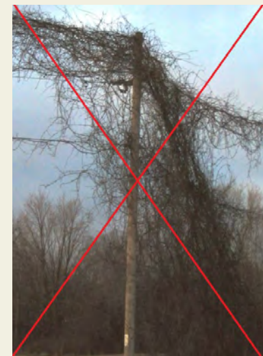
Guy-wire growth contacting electrical equipment & powerlines
