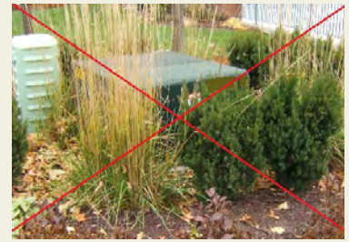
Obstruction around a transformer
