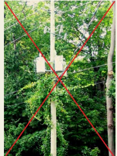
Pole growth contacting electrical equipment & powerlines
